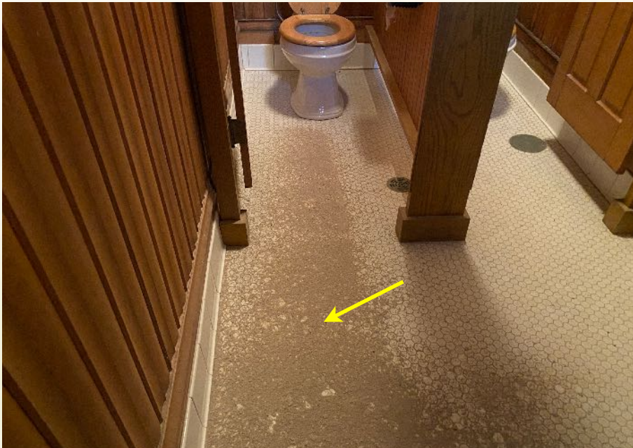
At the restrooms located directly below the limestone stairs and landings we observed a significant amount of limestone droppings on the floor.
